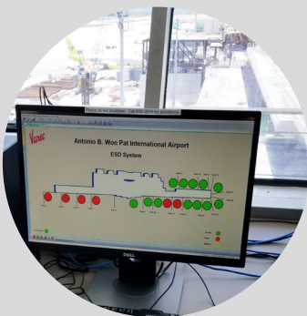
New EFSO System in the Airport Control Tower Running on FuelsManager 10
