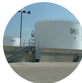
OAL Tanks at Chicago O’Hare Tank Farm
