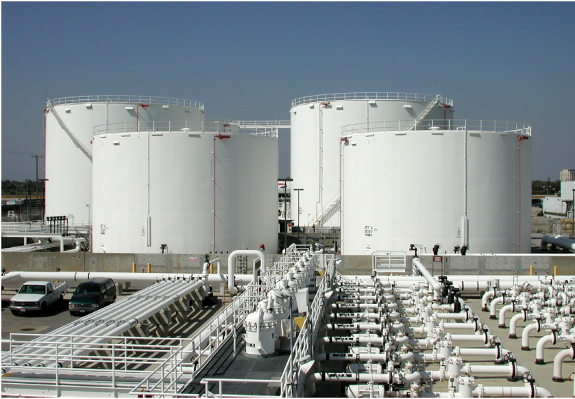
Figure 1. Airport fuel storage tanks and hydrant pumps.
