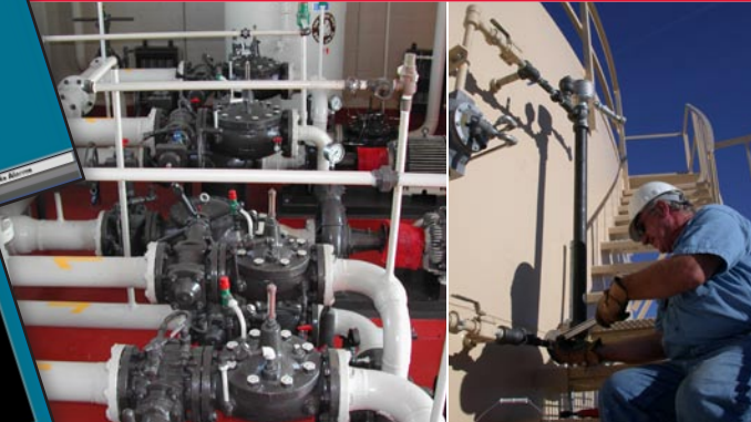
Complete status and critical alarms indications - previously available only on the Control Panels - are now available on the desktop of all authorized FuelsManager users
