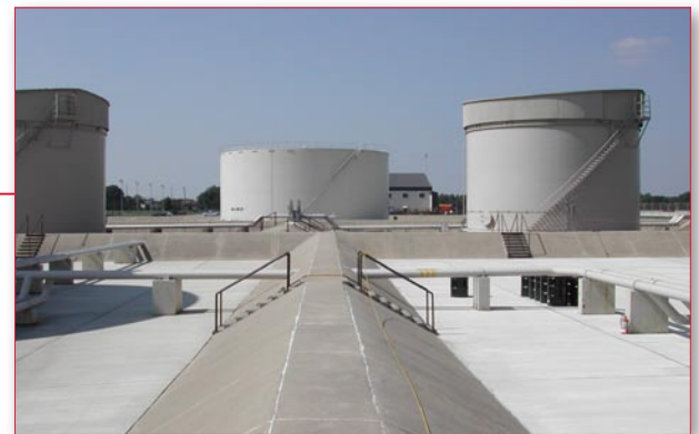
JP-8 fuel bulk storage tanks and hydrant fueling system operated by Liquid Fuels Maintenance (LFM) personnel
